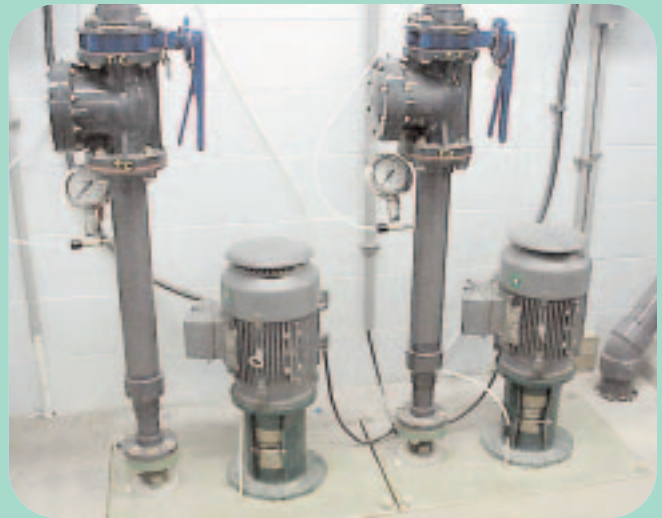
Fybroc Series 5500 Vertical pump installation
