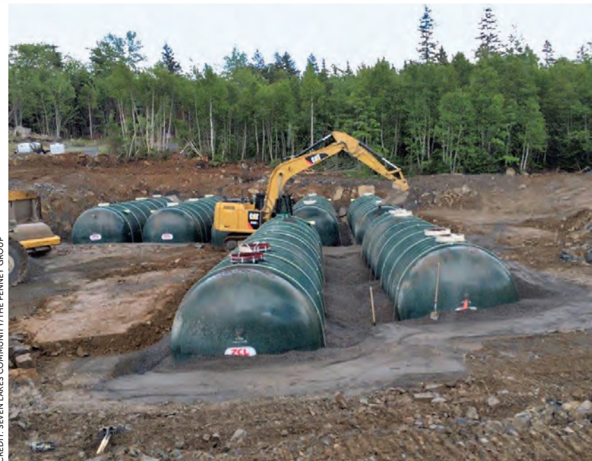
Repeat performance. Massive storage tanks store wastewater until it can be biologically broken down and used to recharge groundwater.
