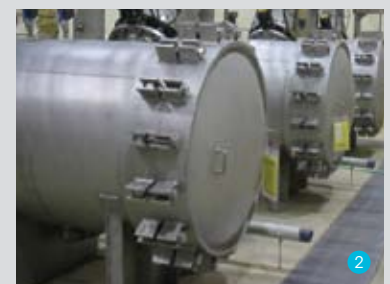
1. DISTRIBUTION MANIFOLD 2. PRETREATMENT
