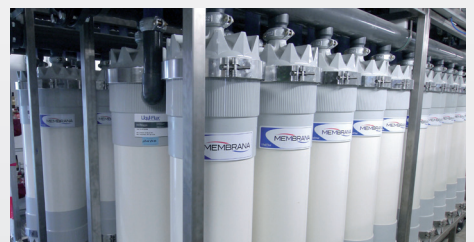
Drinking Water Treatment | 180m 3 /h
