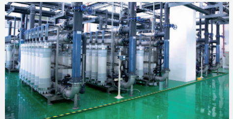
Waste Water Re-use | 1000m 3 /h
