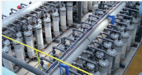
Pre-treatment to Reverse Osmosis | 540m 3 /h
