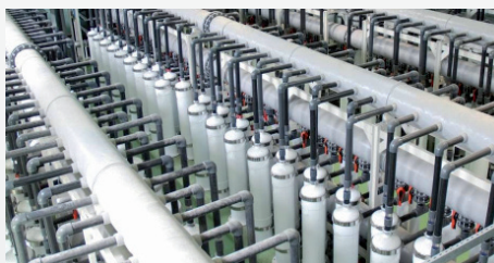
Waste Water Re-use | 2250m 3 /h
