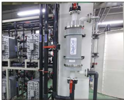
10-inch Oxygen Removal System
