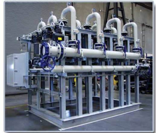
14-inch Boiler Feedwater System
