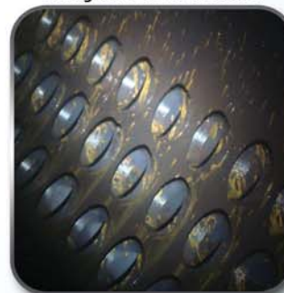
Pitting In Boiler Metal Surface
