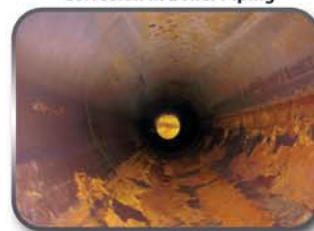
Corrosion In Boiler Piping
