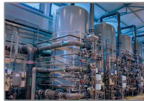
Mixed Bed Demineralizer for a Power Generation Facility
