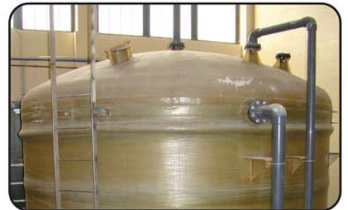
Chemical Storage Tank
