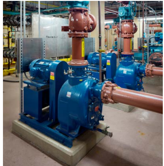
Super T Series® pumps in the basement of a sludge loading application
