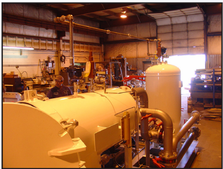
Fuel Transfer Skid
