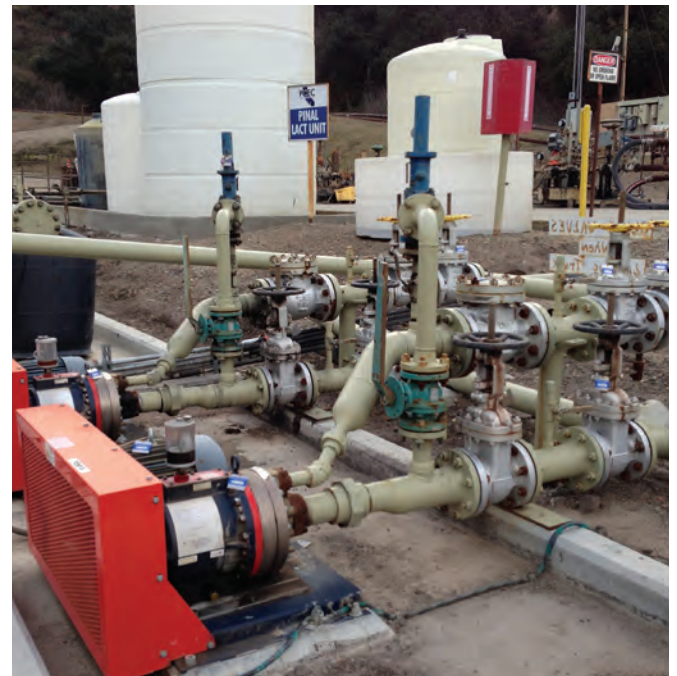
Hydra-Cell pumps shown processing volatile crude oil.
